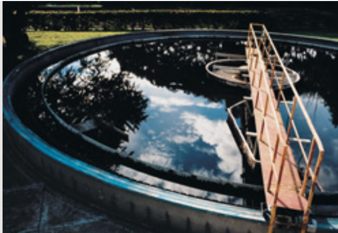
Left: The water treatment plant in Bugalagrande, Colombia has won many awards.
