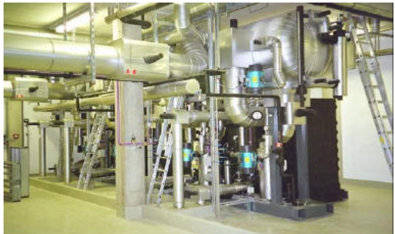
CO 2 condensers - NH 3 evaporators in the plant room
