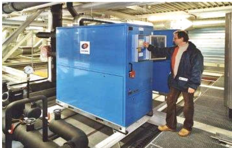
Water chiller with an ammonia charge of less than 4 kg
