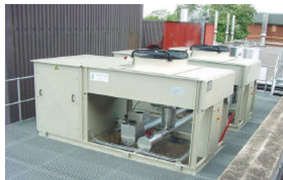
Hydrocarbon water chillers
