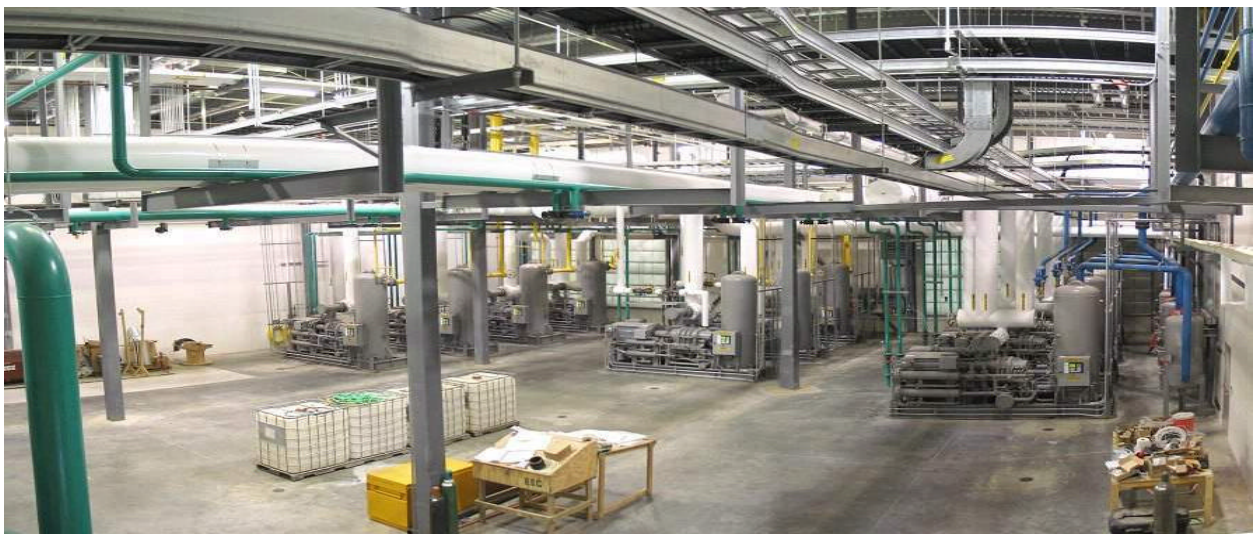
Largest CO 2 plant in the world at Jonesboro – USA
