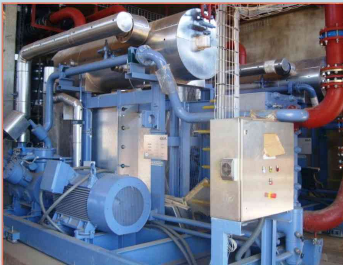
Chillers at Flowergate Factory
