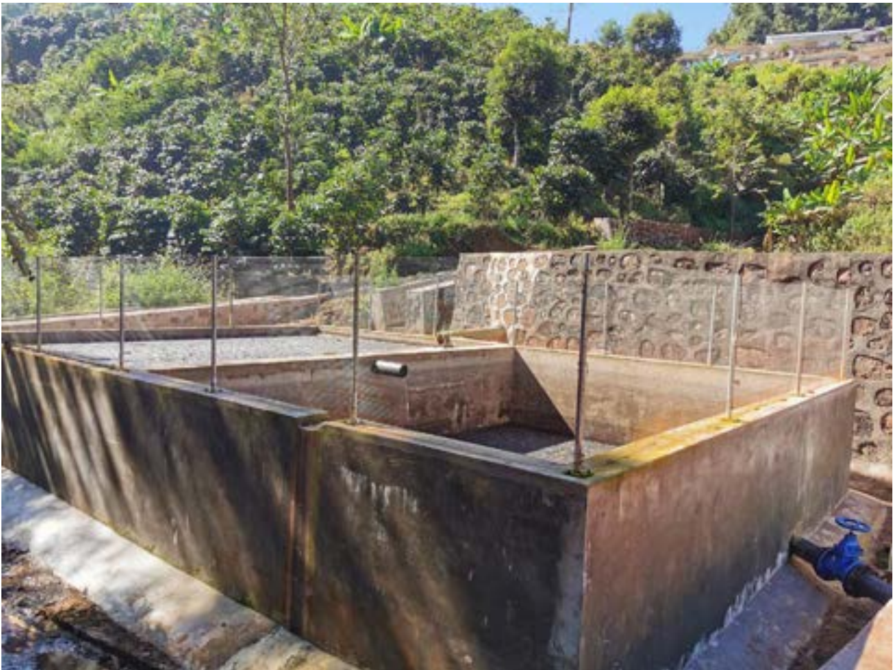
Wastewater treatment tank | Nestlé.
